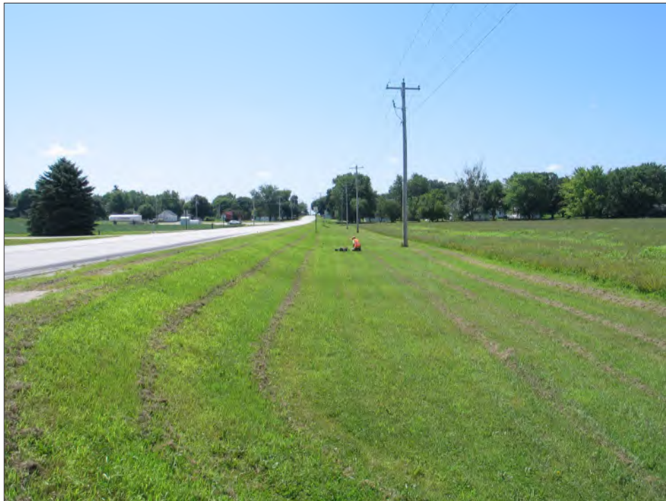
Figure 19. Water main replacement corridor at the intersection of Fitzpatrick and Adrian streets. View to the south (7/15/25).
