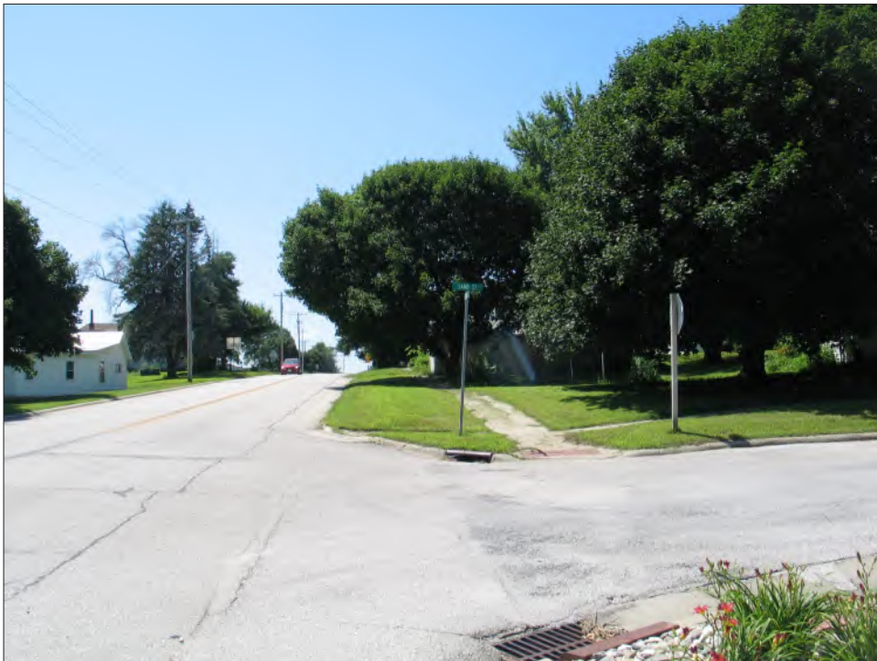
Figure 17. Water main replacement corridor at the intersection of Fitzpatrick and Sand streets. View to the south (7/15/25).
